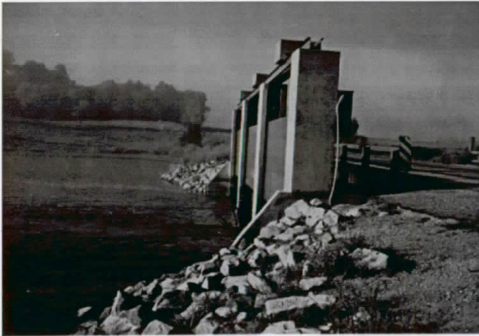
Figure 1. The flood control gates installed on the inlet/outlet channel between Lake Poinsett and the Big Sioux River.
