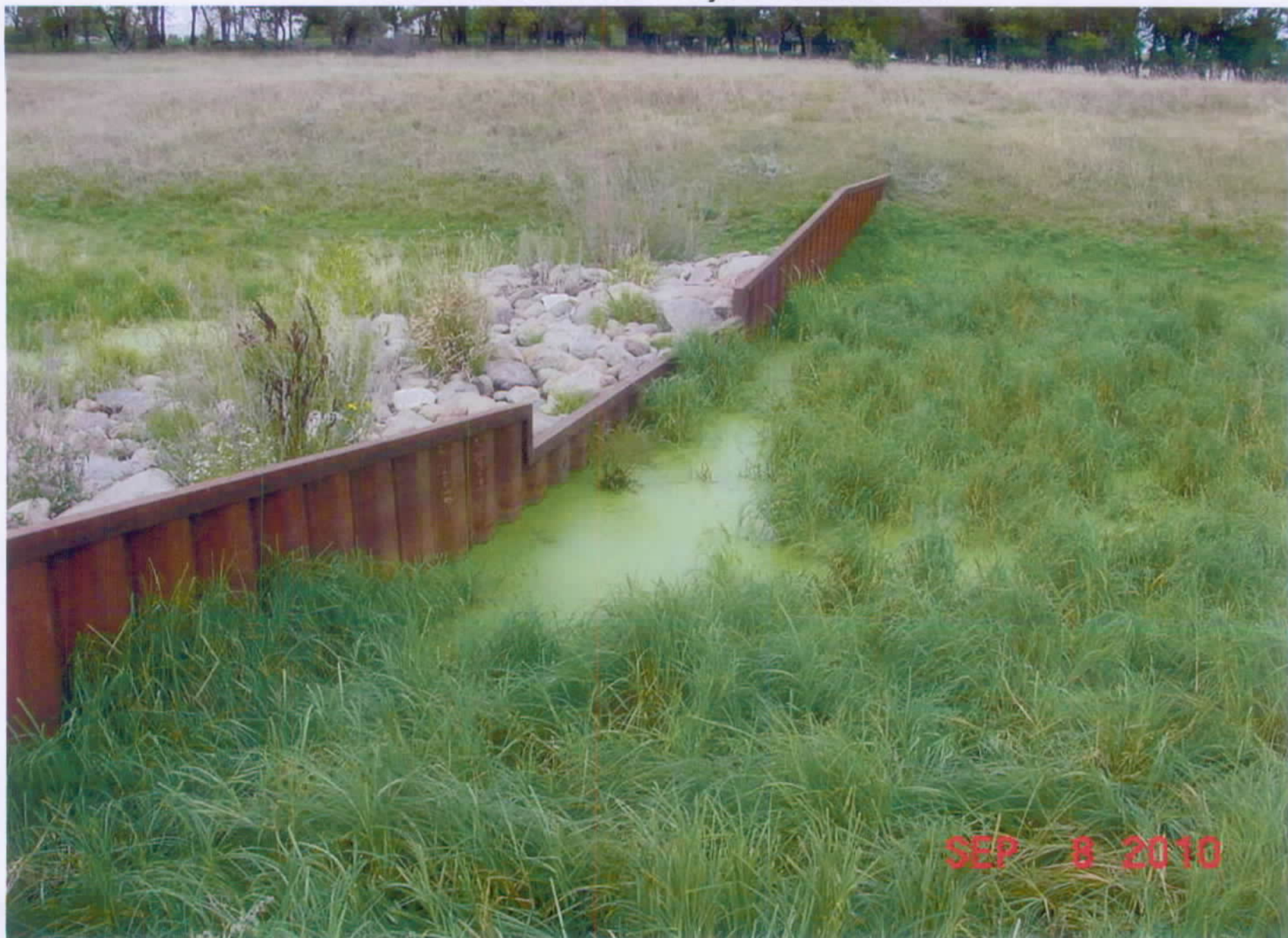
Lake Pelican Water Project District Weir
