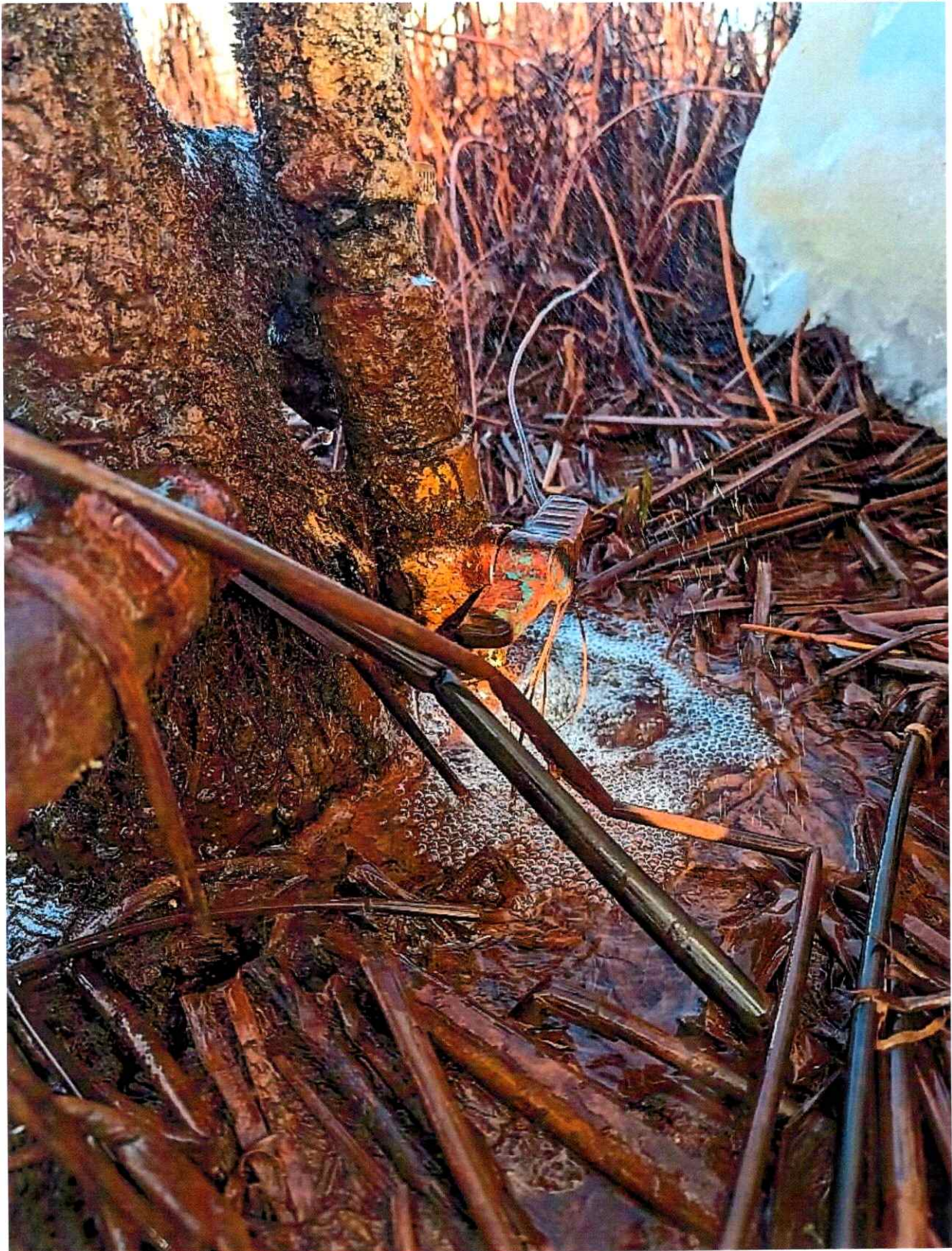
Water Flowing from Valve
