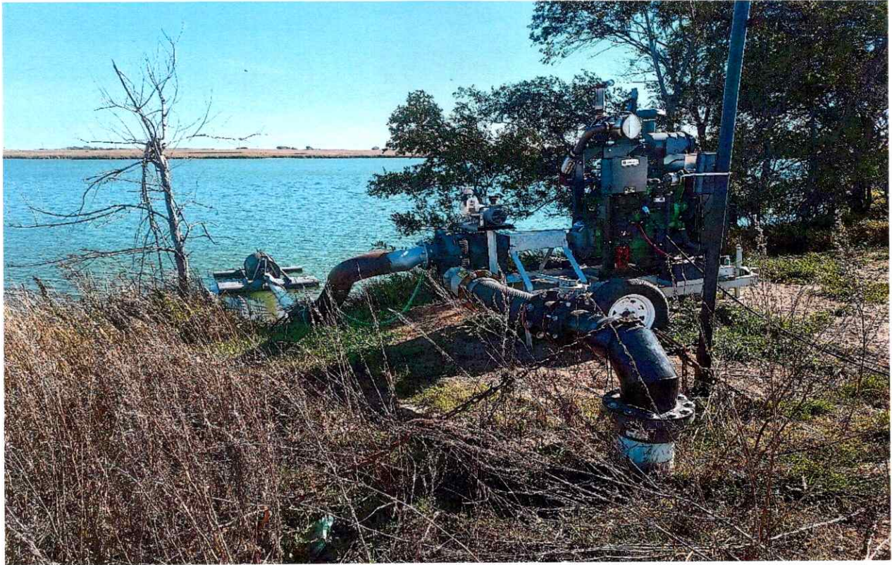
Pumping plant located on Reetz Lake in Day County.
