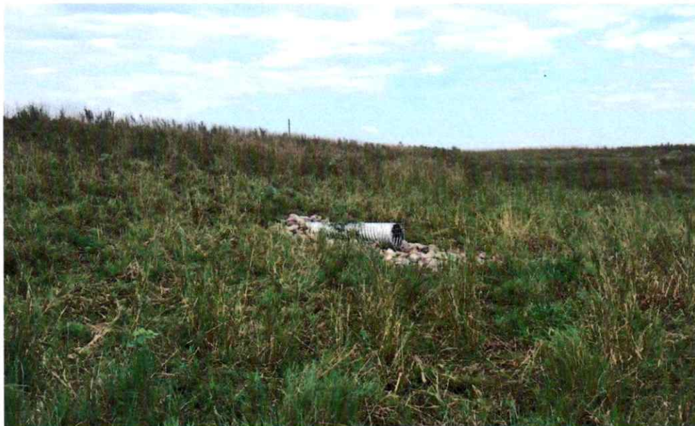
PIC 4. Looking north at the 24-inch primary outlet discharge pipe. Note: the soil was saturated indicating seepage through and under the dam.
