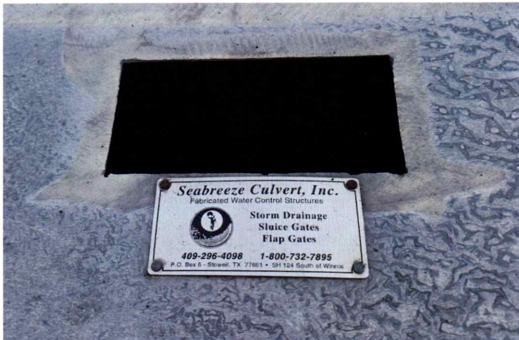
PIC 3. Primary outlet technology using a Seabreeze water control structure to maintain a specified depth in the pond.
