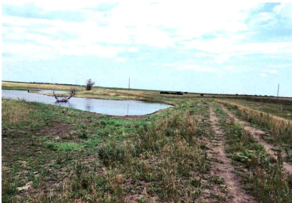
PIC 2. Looking north along the centerline of the dam with poor to fair vegetative cover.
