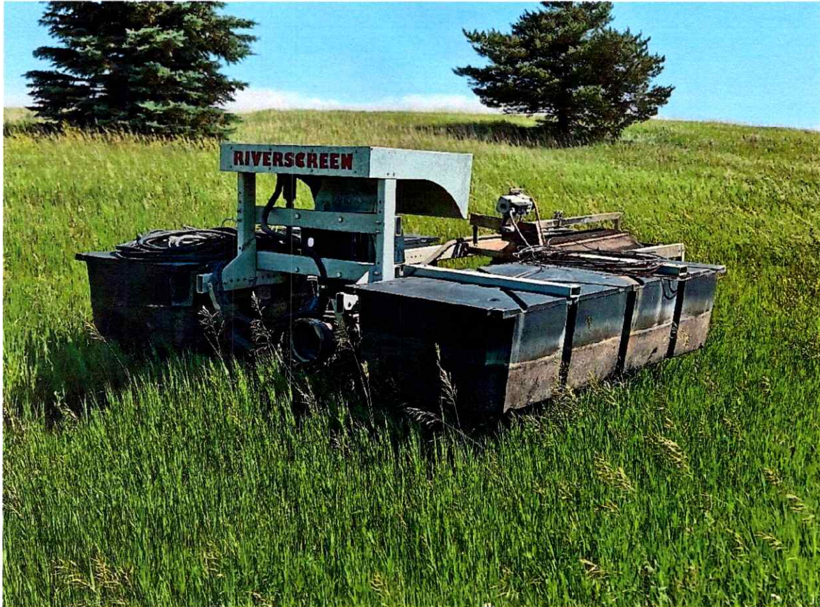
James River floating platform pumping plant.
