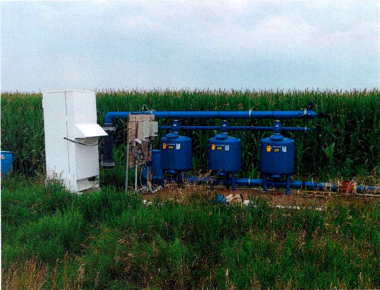
Sand filters used to treat well water for the subsurface drip irrigation system. The well is located to the left of the white box.
