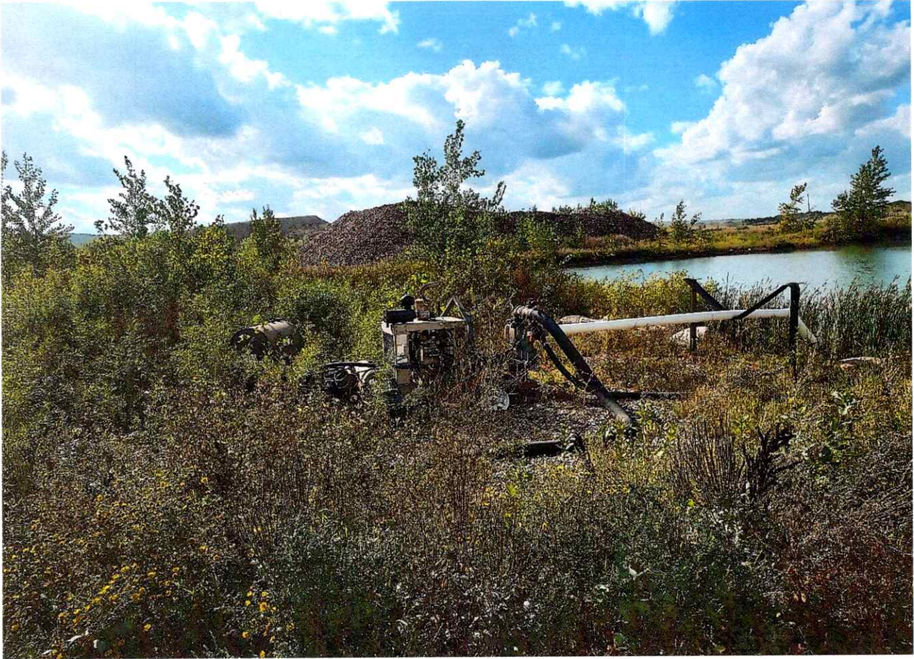
Power unit and pump used to take water from a surface pond and transport it to a wash/sediment pond.
