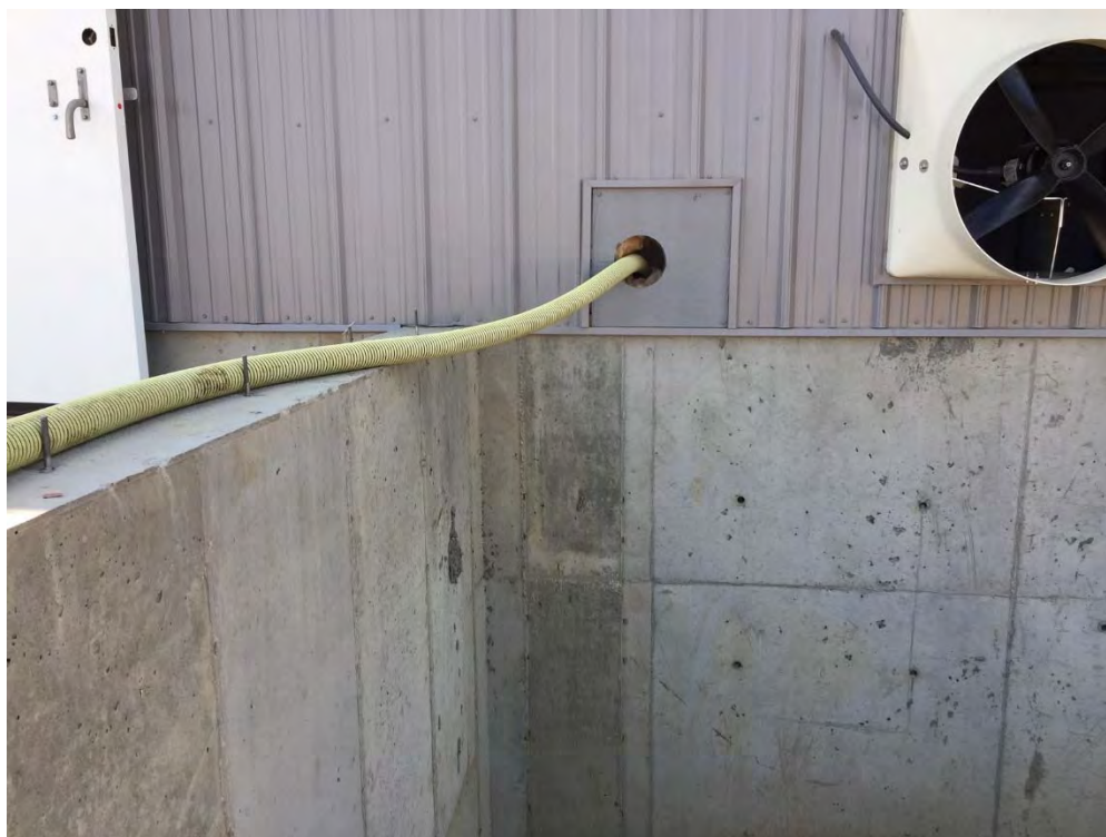
Photo 8: Well #1 discharge hose enters barn containment area (looking west).
