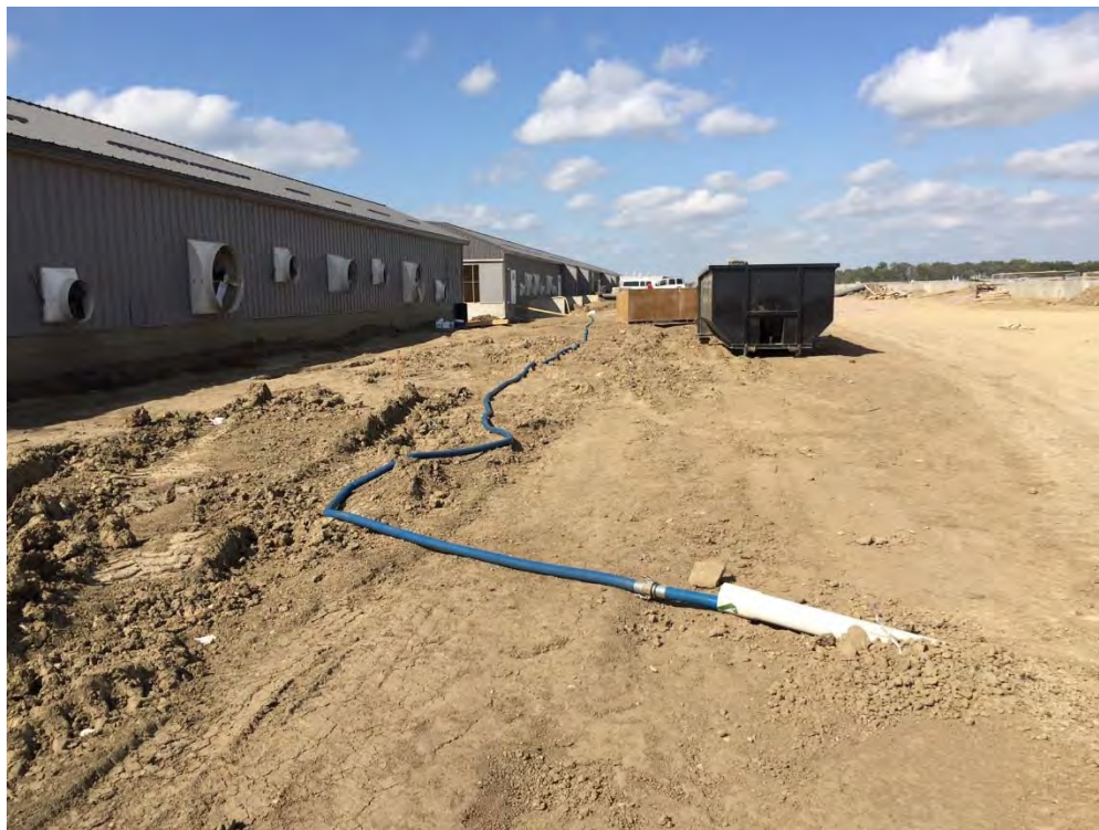
Photo 7: Well #1 discharge hose looking north.
