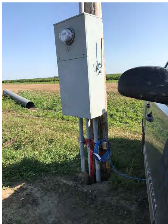
Photo 10: Barotroll attached to nearby power pole.
