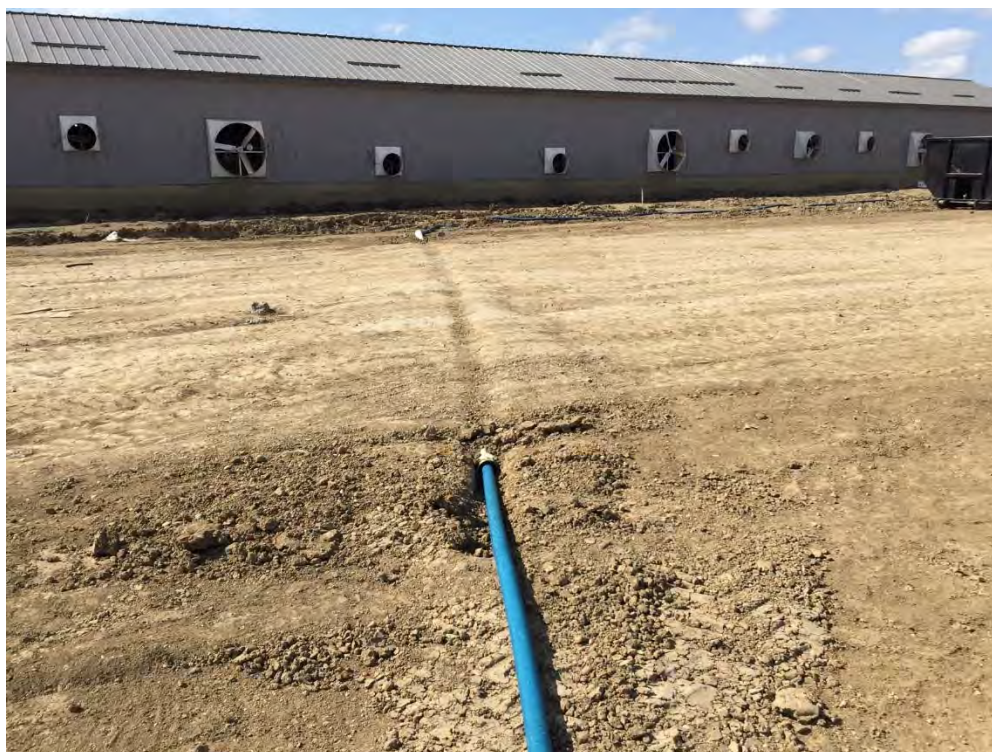
Photo 6: Well #1 discharge hose looking northwest.
