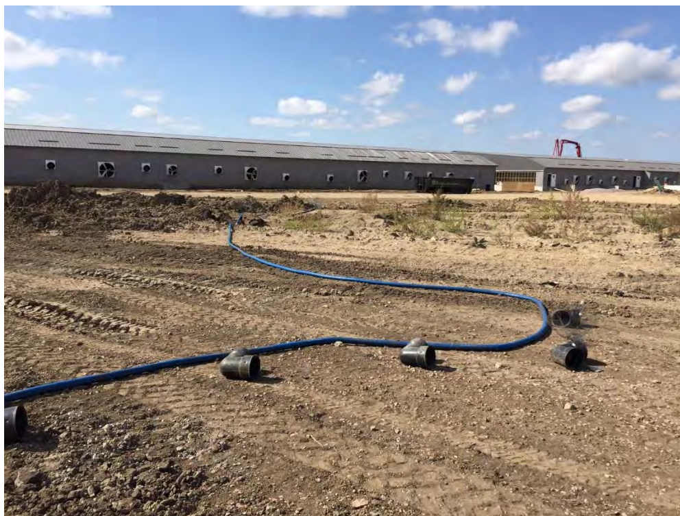
Photo 5: Well #1 discharge hose looking northwest.
