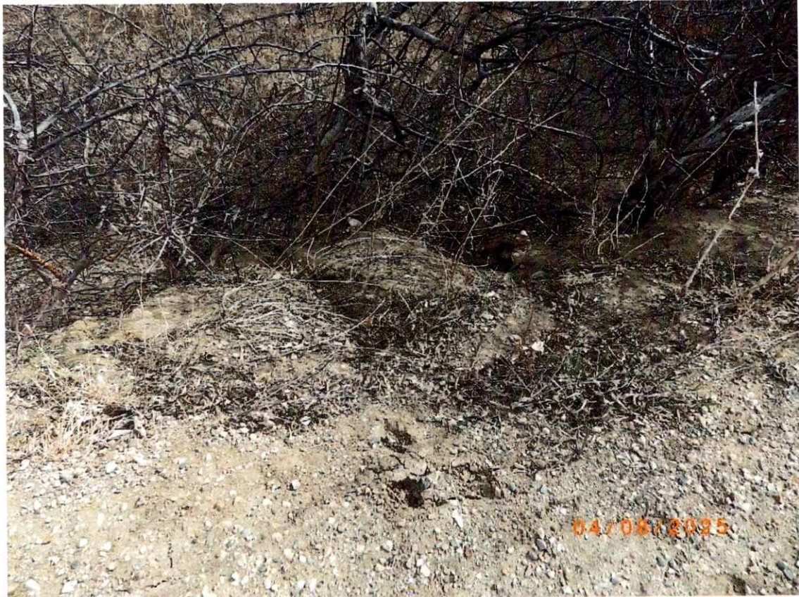
Example of erosion on the downstream slope.
