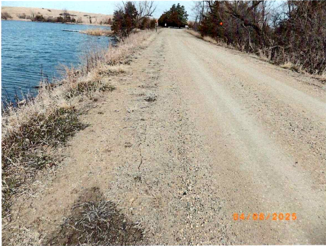
Crest and upstream slope. Note area of cracking.
