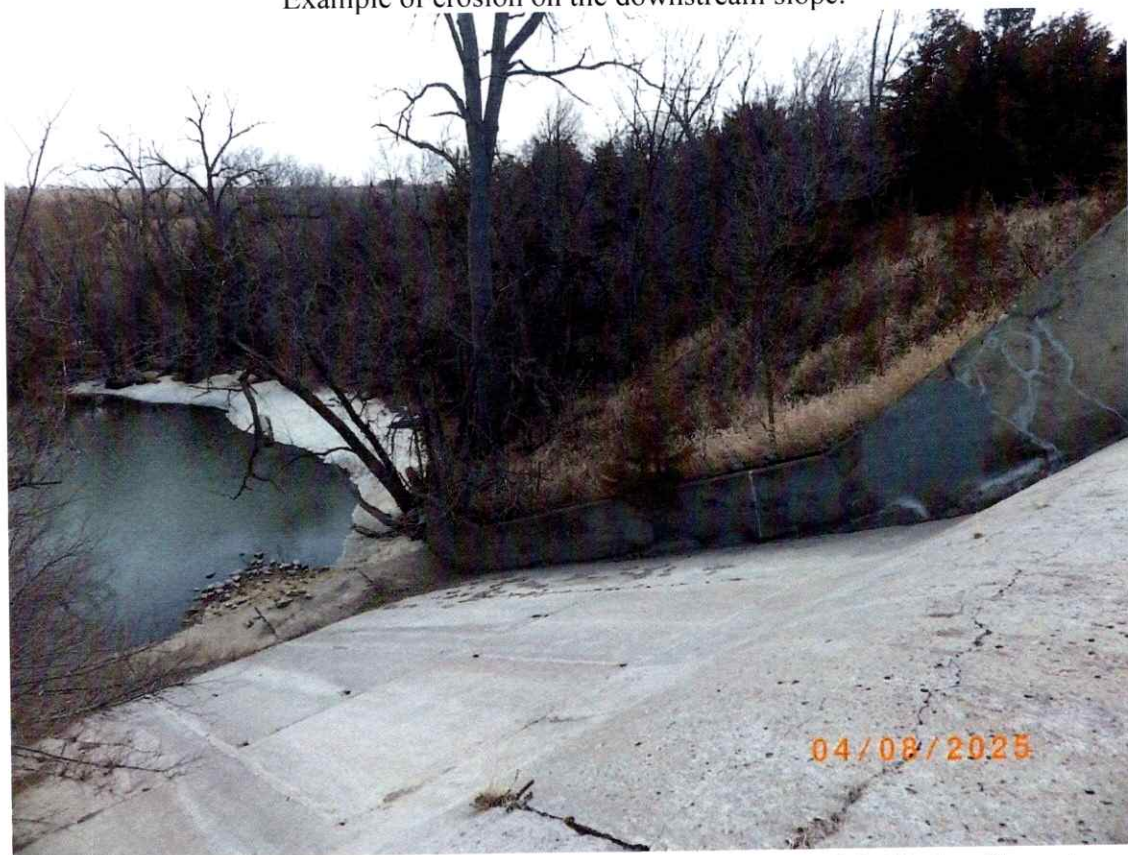
Primary spillway. Note plant growth in joint, ponded water at tow, tree growth behind walls, and cracking.
