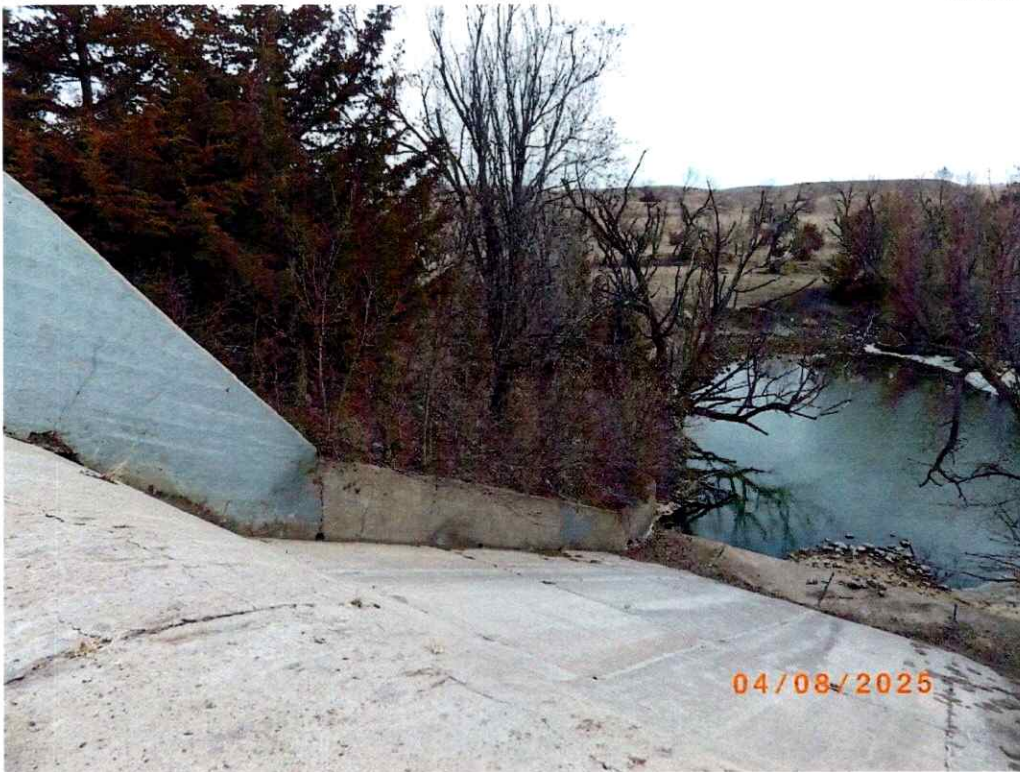
Primary spillway. Note spalling along base of the left wall.
