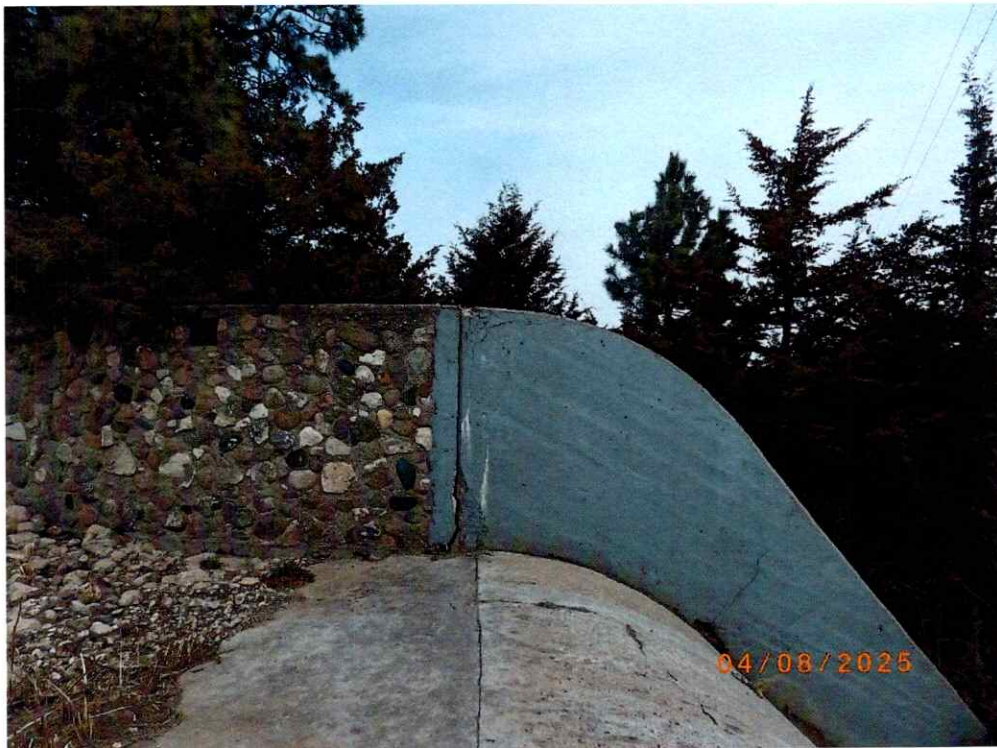
Primary spillway. Note dirt at wall drain. Dirt is visible in crack/separation between cobble stone approach wall and concrete spillway wall.
