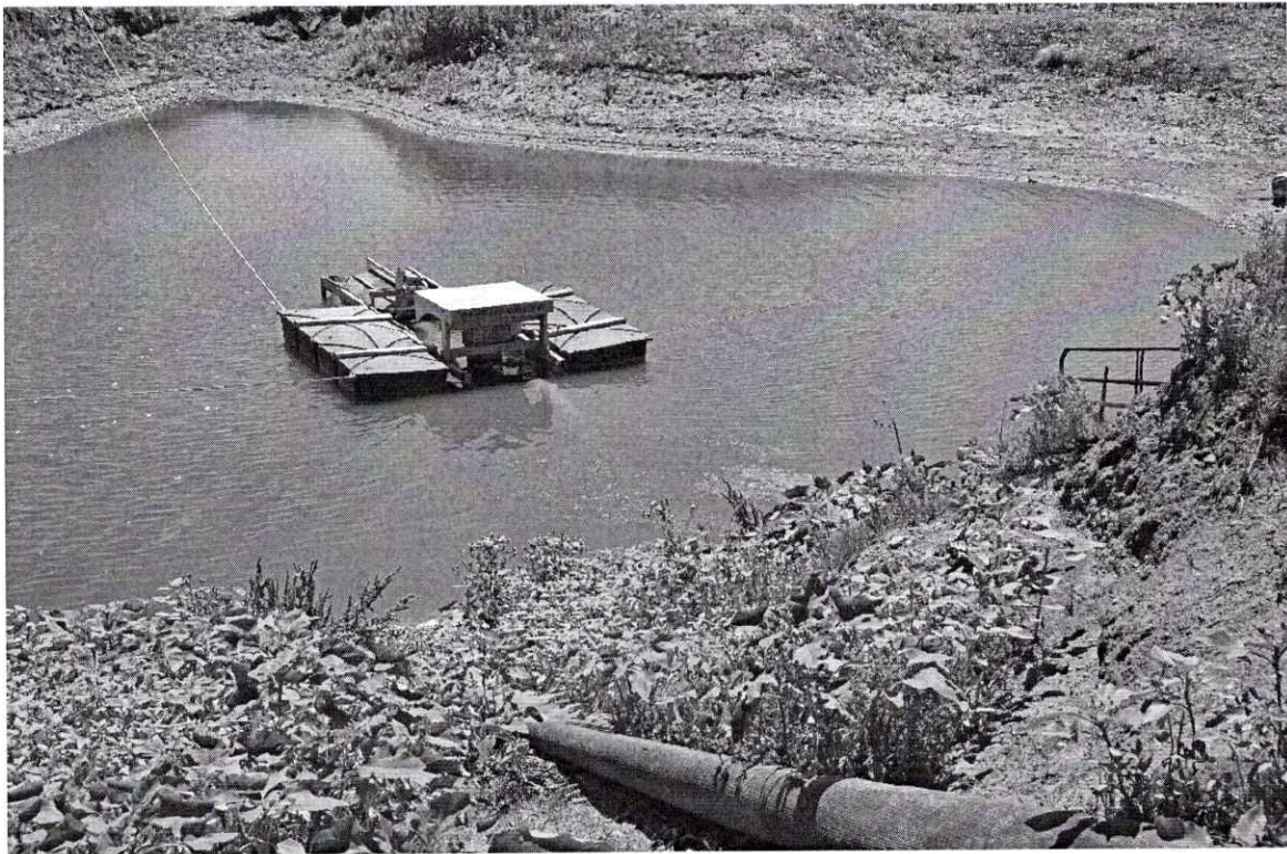
Permit 8166-3 Gravel pit pumping plant.
