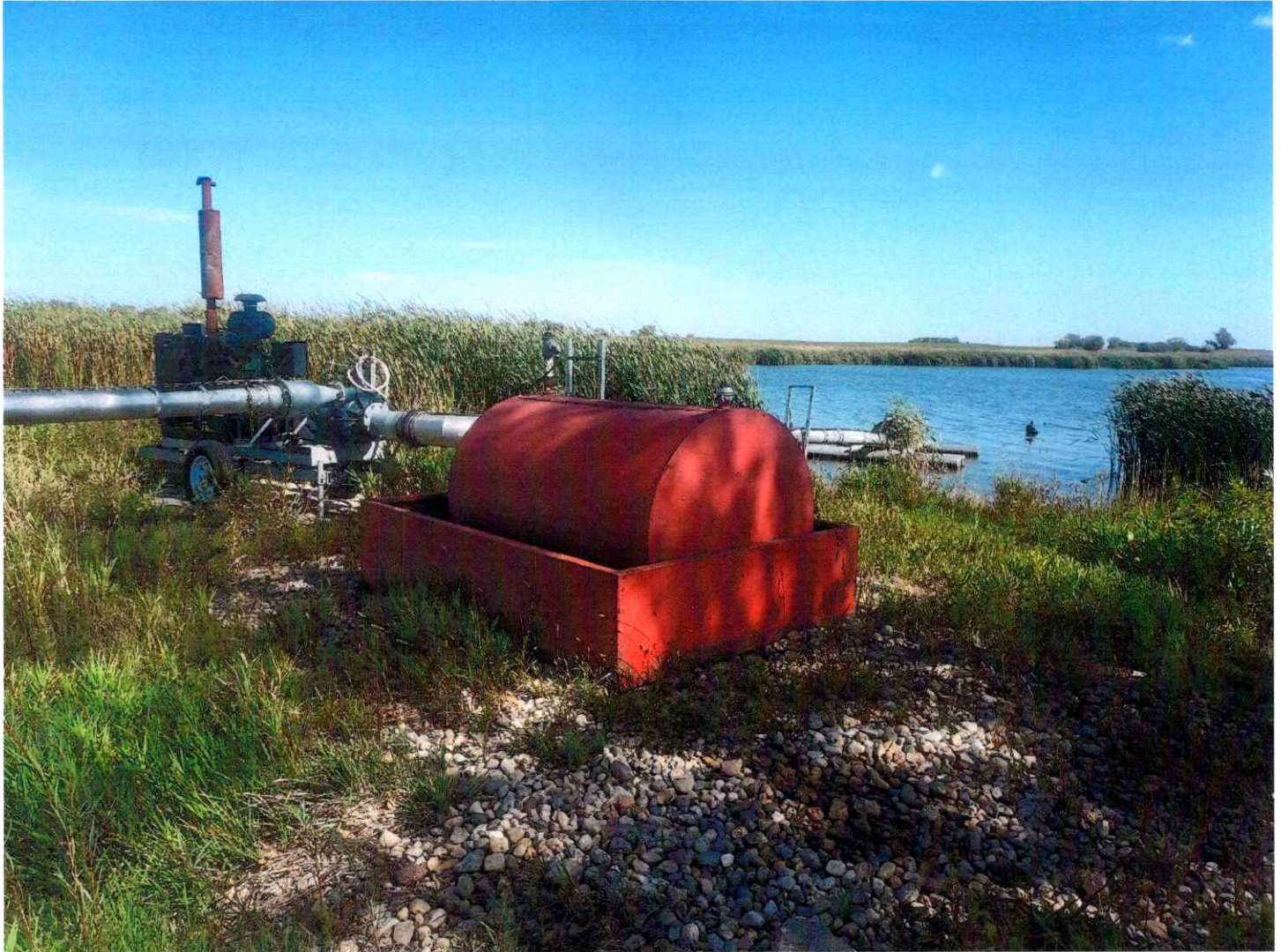
PUMPING PLANT AT ANTELOPE LAKE
