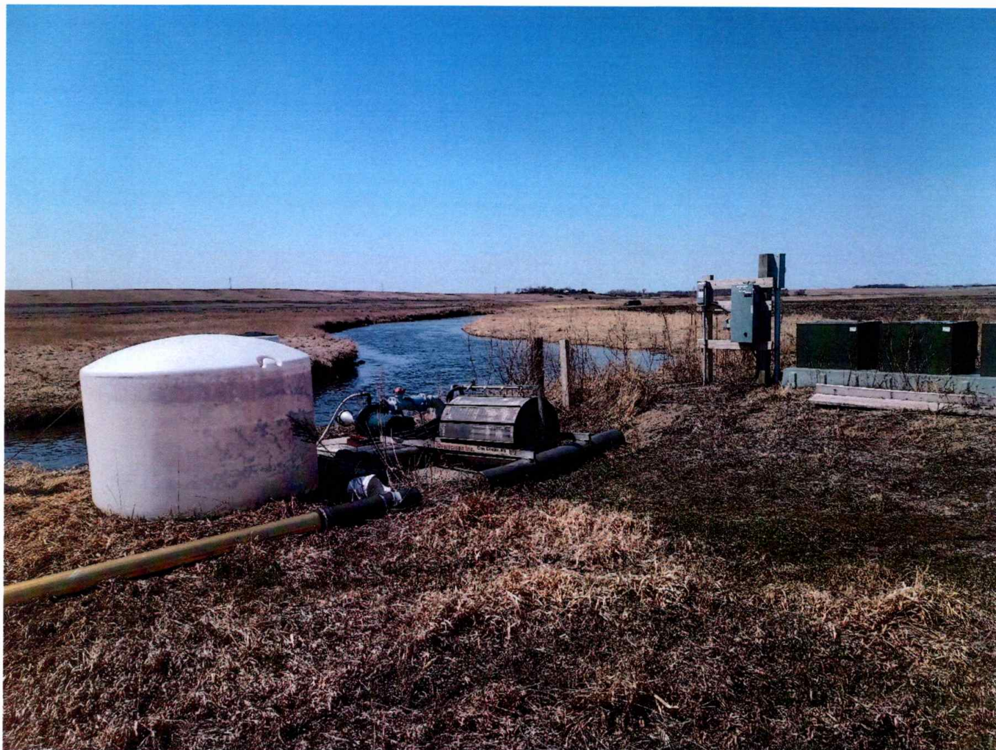
Pumping plant on the bank of the Big Sioux River.
