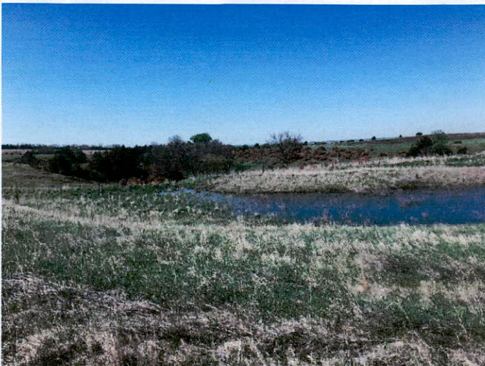
Looking South Southwest at the Overflowing Auxiliary Spillway.
