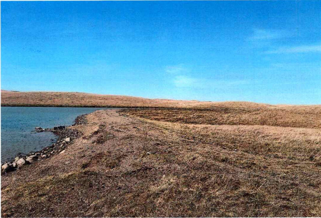
PHOTO #1. Looking northwest along the dam crest showing no vegetation on the crest due to cattle traffic. Also, there is no vegetation on the upstream side of the dam as this is where cattle access the water for drinking purposes. Note the curvature of the dam and the location of the principal outlet spillway.
