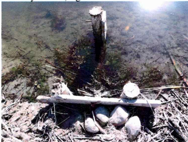
Figure 1 – plugged outlet tube.
