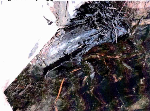
Figure 2 – debris removed from the outlet tube.
