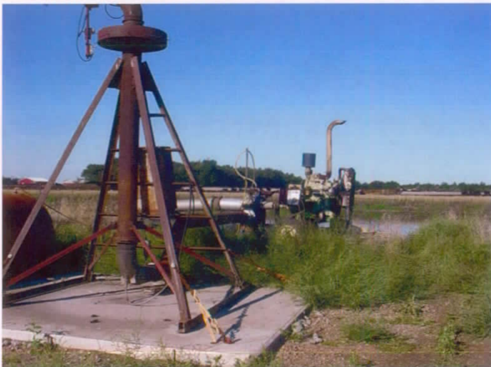
Diesel motor and pivot next to wastewater lagoon as in place on September 10, 2007
