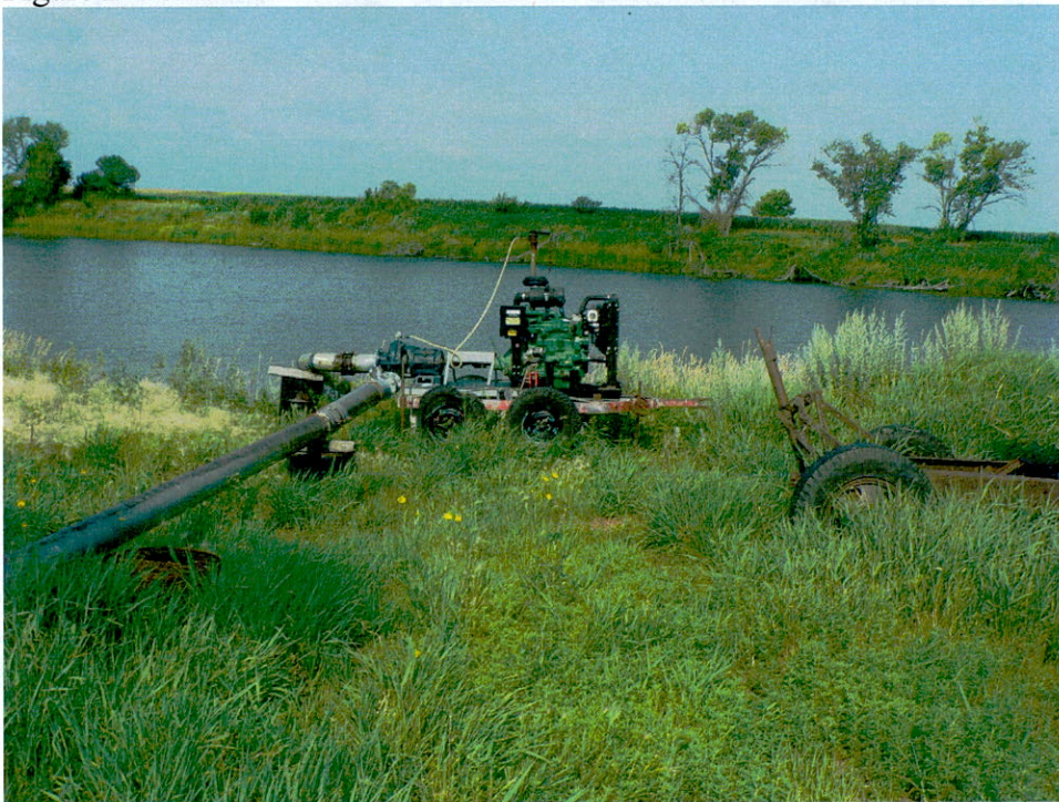
Figure 3 – Pump, motor and intake located in SW¼ of Sec 10 T114N-R62W
