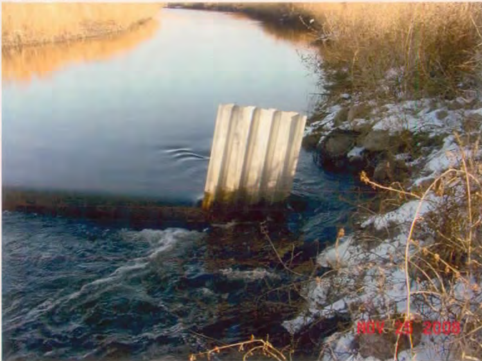
November 2008 - Erosion around south end of outlet at the Putney outlet structure SW \frac{1}{4} Sec 18 T124N-R62W
