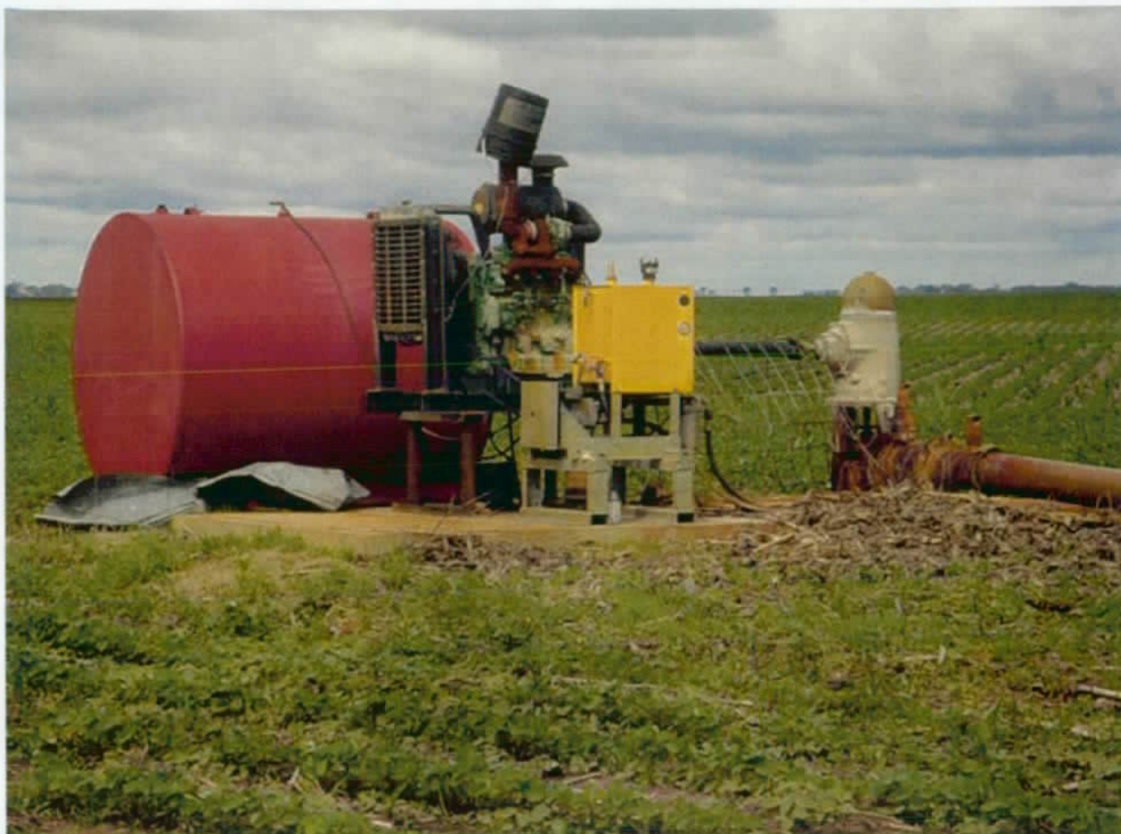
Well, motor, and fuel tank at pivot point for Water Permit No. 6196-3 - pivot point is located approximately 150 feet northeast of well.
