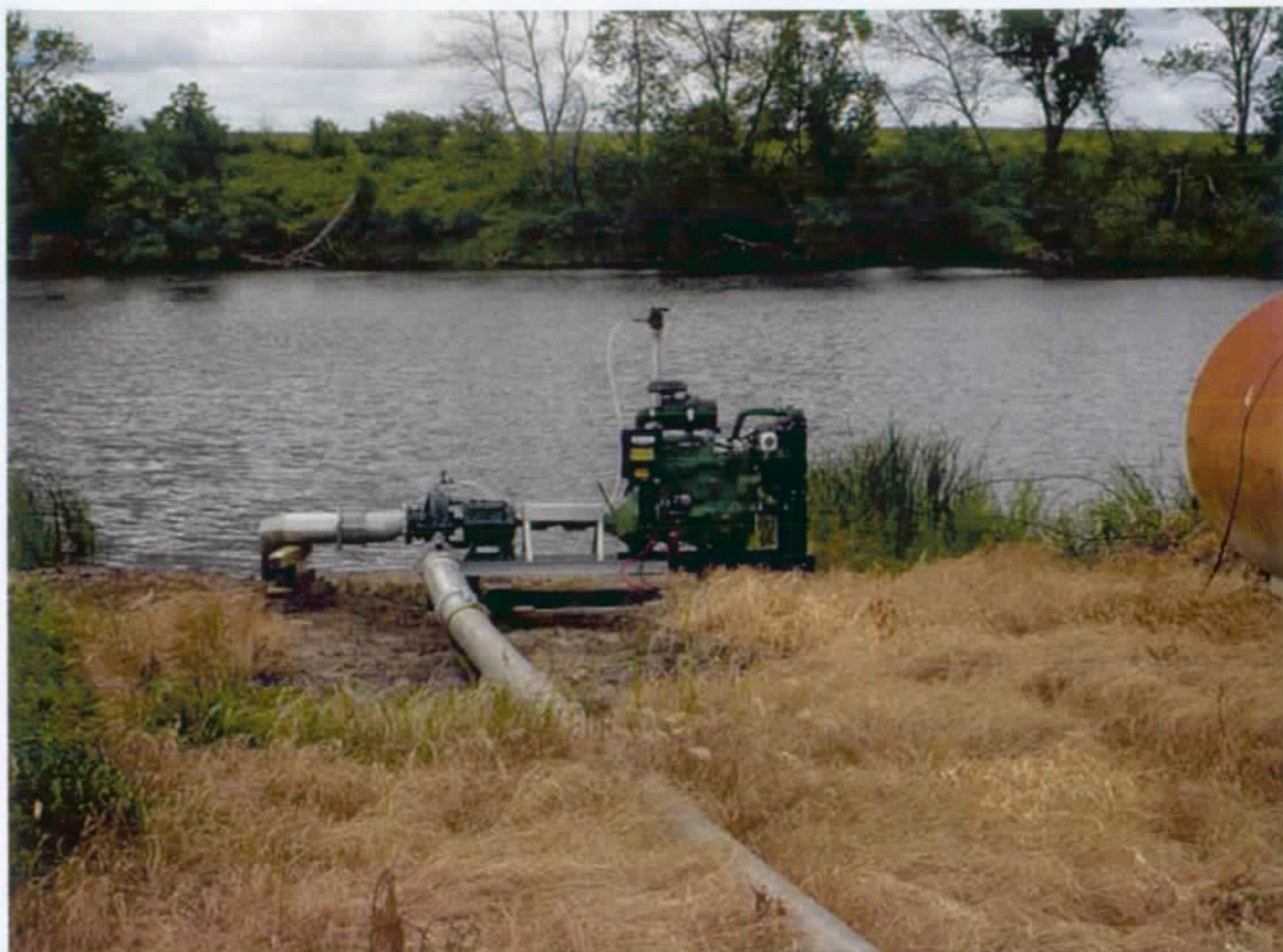
Pump site No. 4 located in the SW \frac{1}{4} SW \frac{1}{4} Section 10, T114N, R62W
