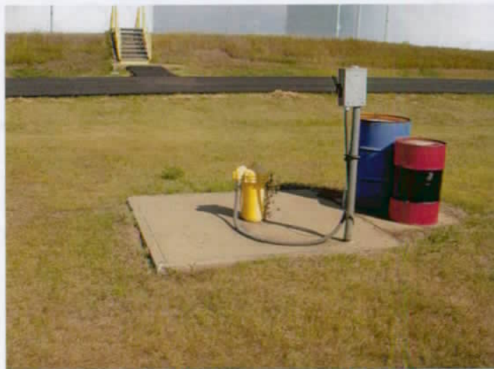
Secondary well (authorized by Water Right No. 2972-3 and used only for emergency purposes)
