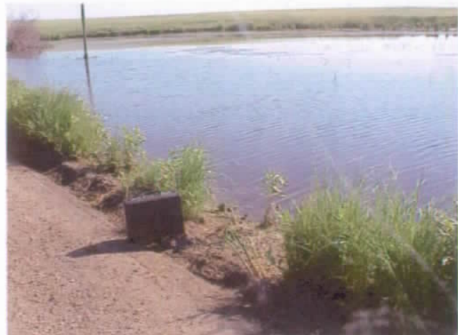
A6: Road crown about 1 foot above water near corners of sections 35, 36 and sections 1, 2
