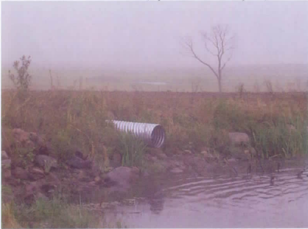
Inlet to 24 inch culvert acting as primary spillway on the east side of the dam embankment. Pool elevation is 18 inches below bottom of culvert.
