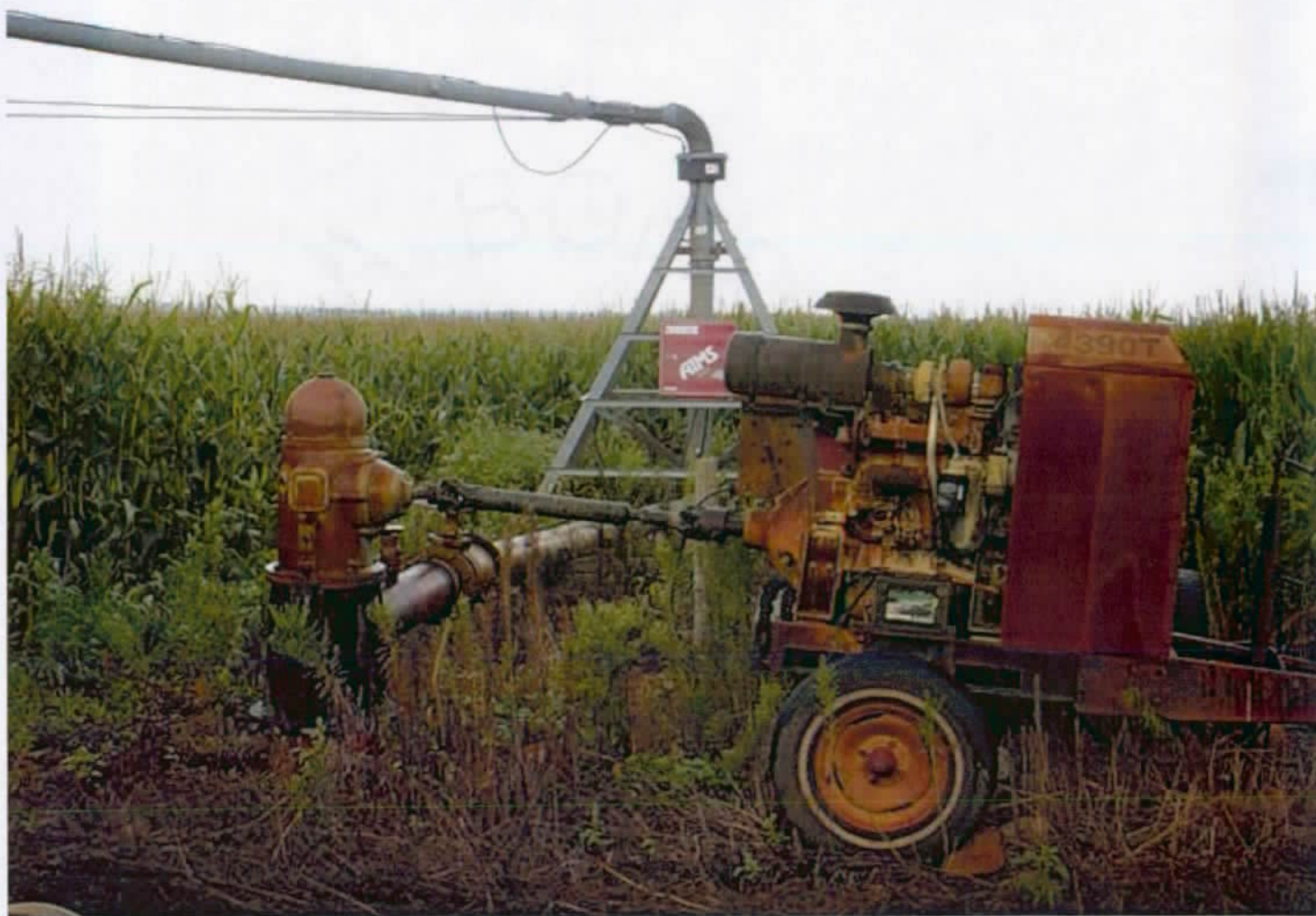
Water Permit No. 5899-3, Tim Ostrem – well, motor and center pivot
