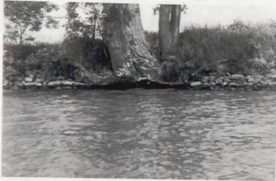
PHOTO NO. 5 Tree on Island Destruction Line Elevation---1252.9
