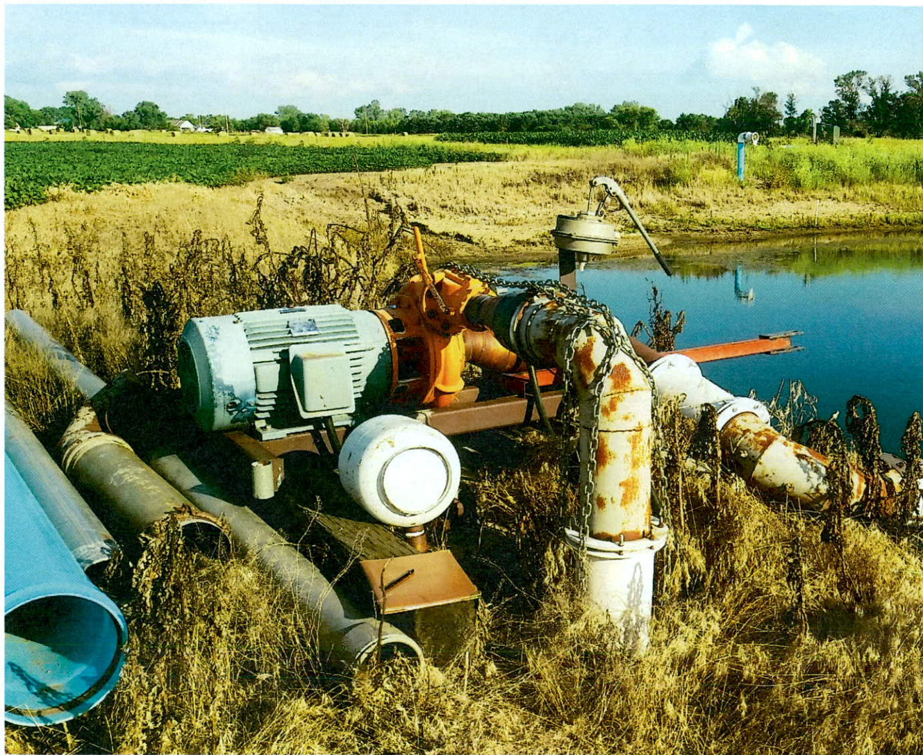
Picture 5. Marathon electric motor and pump in foreground with standpipe outlet for water pumped from Froning pond shown in upper right-hand corner of picture.
