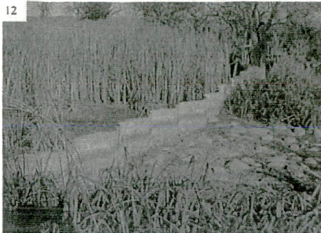
10-17-00 - Sheet pile outlet low elevation 1827.4 fmsl.
