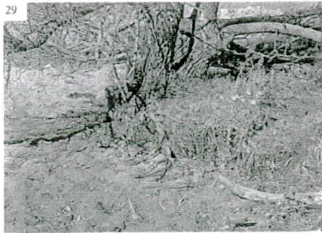
10-18-00 - Multi trunk ash lk side 1828.5 and ld side 1829.1 fmsl; top of erosion 1828.5 fmsl.
