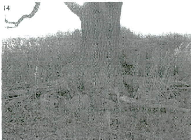
10-17-00 - 3.5' dia. ctw lk side 1828.4 and ld side 1831.1, top of washed roots 1830.1, bottom of erosion 1829.0, and top of erosion 1830.4 fmsl.
