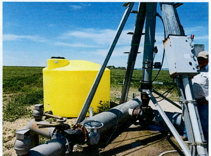
Appurtenances at south 156 ac. pivot with incoming 10" line from irrigation district and outgoing line to north pivot (bottom foreground)
