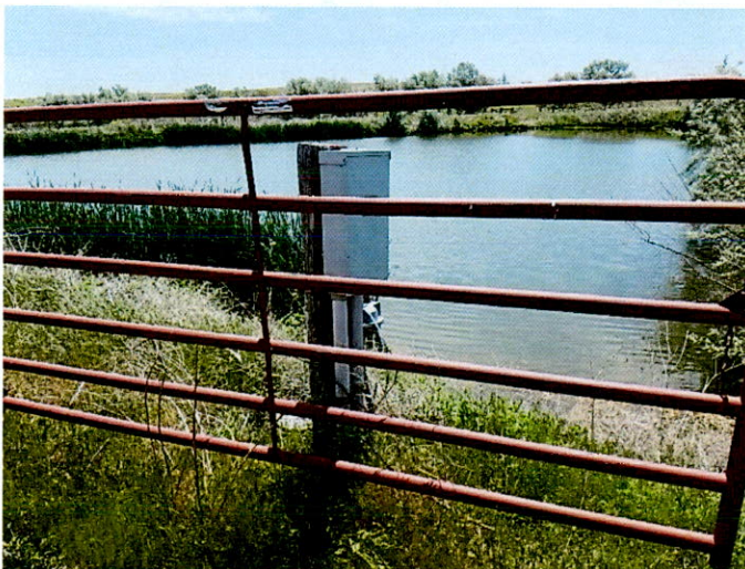
Electrical power for floating inlet and pump
