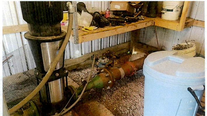
Booster pump at golf course
