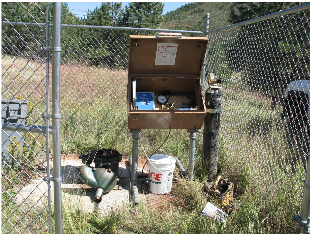
Figure 4. Automated data recording set up at Well No. 2.
