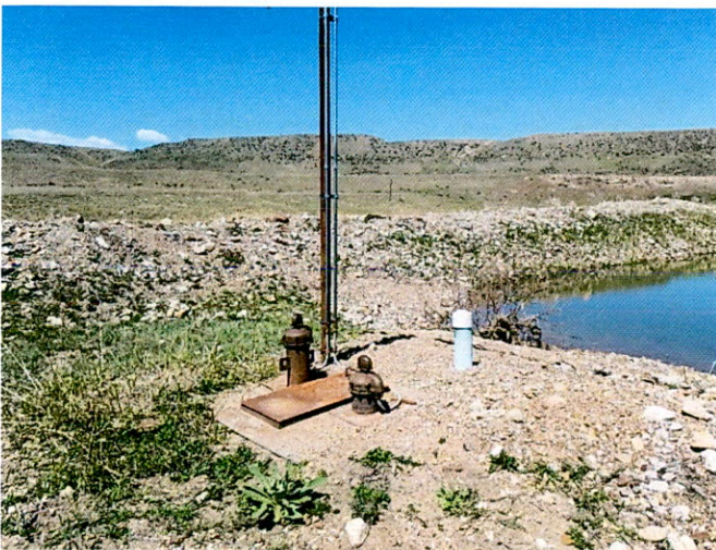
Intake gallery and submersible pumps
