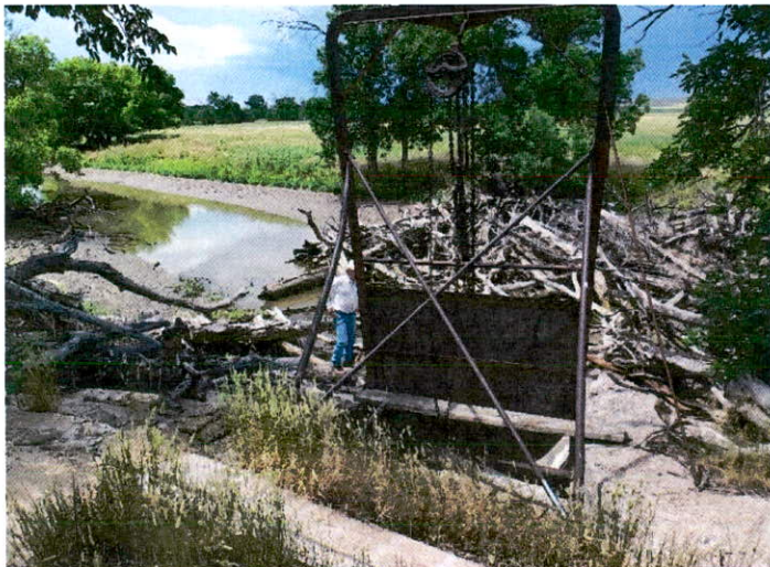
Hoist operated Head gate at Spring Creek Diversion
