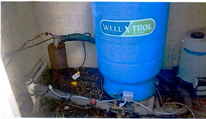
Well #2 (left of pressure tank)
