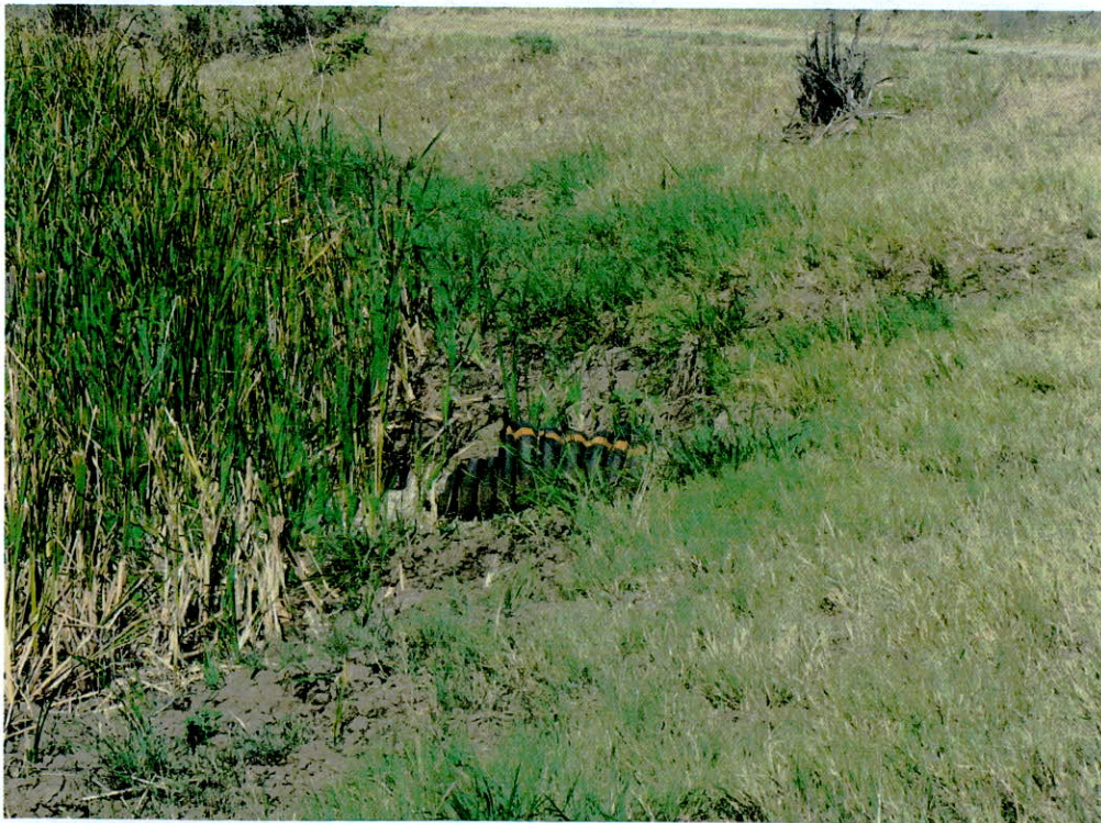
Figure 3 - Photo Location A- Creek flow bypass pipe through the diversion dam on Coal Creek located in the NE \frac{1}{4} NE \frac{1}{4} of Sec 26 T10S-R2E.
