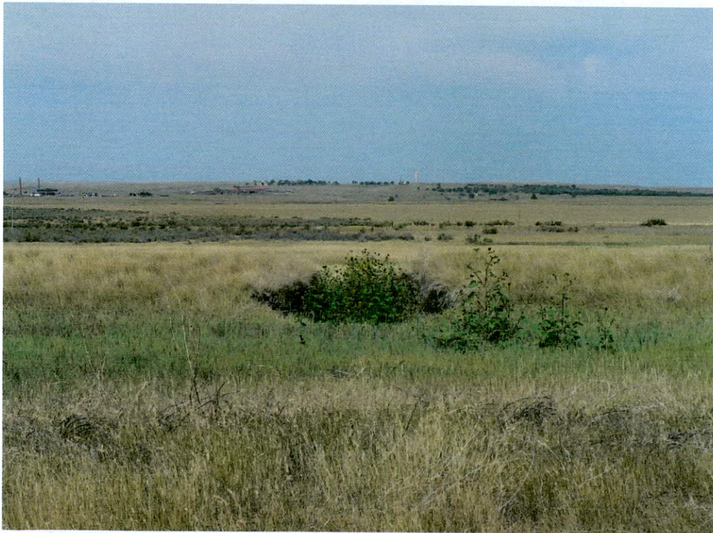
Figure 11 - Photo Location H - A dike breach to the main ditch/dike located in the NW \frac{1}{4} SE \frac{1}{4} of Sec 13 T10S-R2E.
