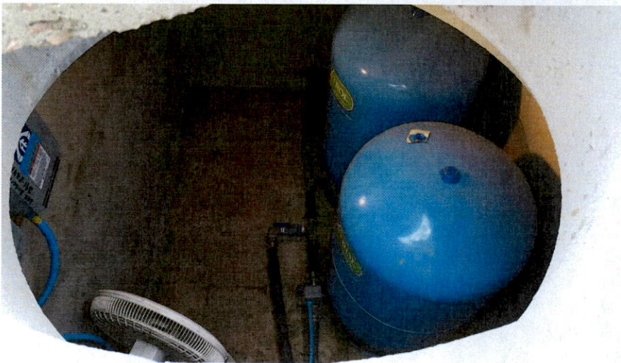
Pit with pressure tanks and controller
