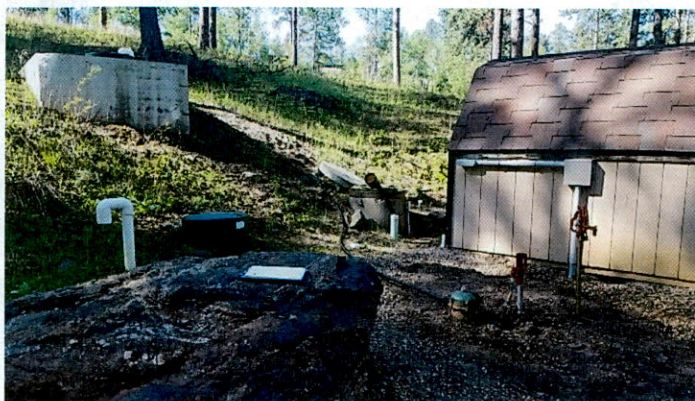
Well #1, pump house, manholes for storage tanks and settling basin (upper left)
