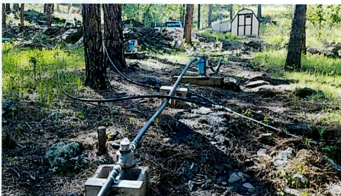
Water meters and filters
