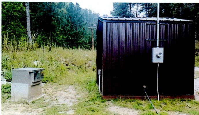
Well # 5 and pump house, well head is located under locked box on left of photo (security)
