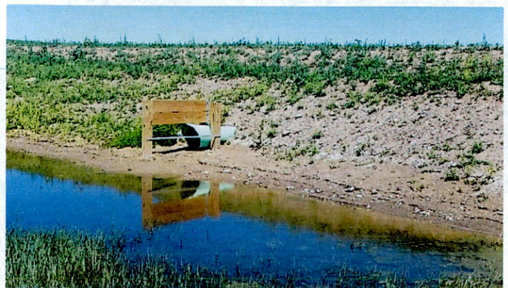
Principal Spillway inlet and anti-vortex/trash rack
