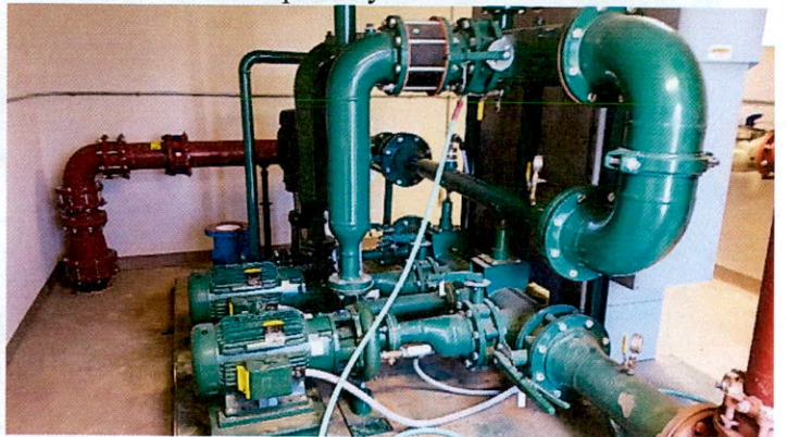
Booster pumps for city supply
