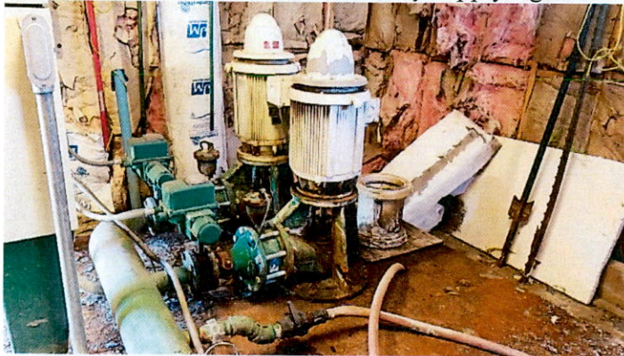
Pumps for pond supply
