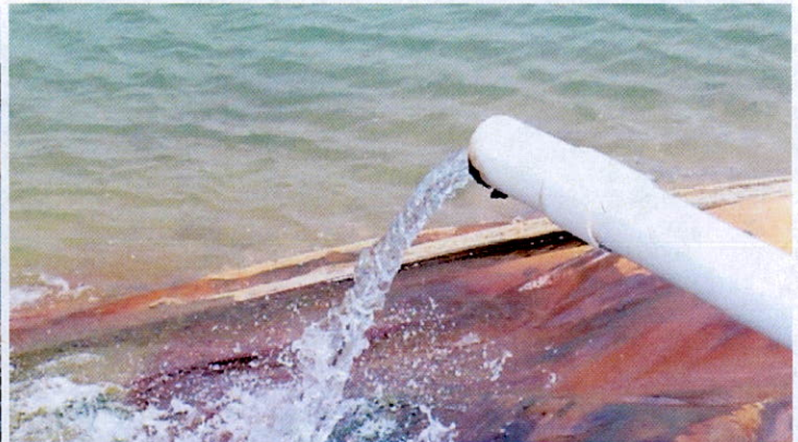
3" PVC inlet to storage pond
