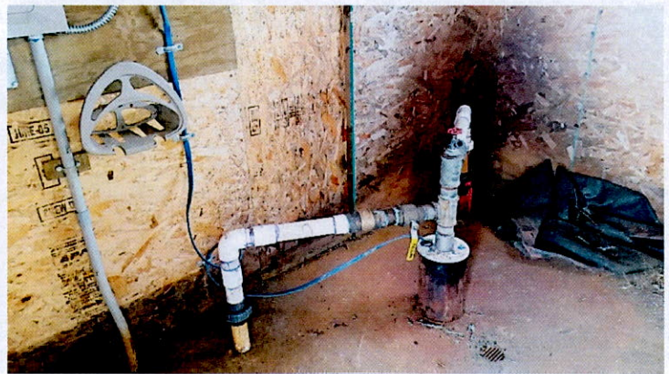
Well in pump house
