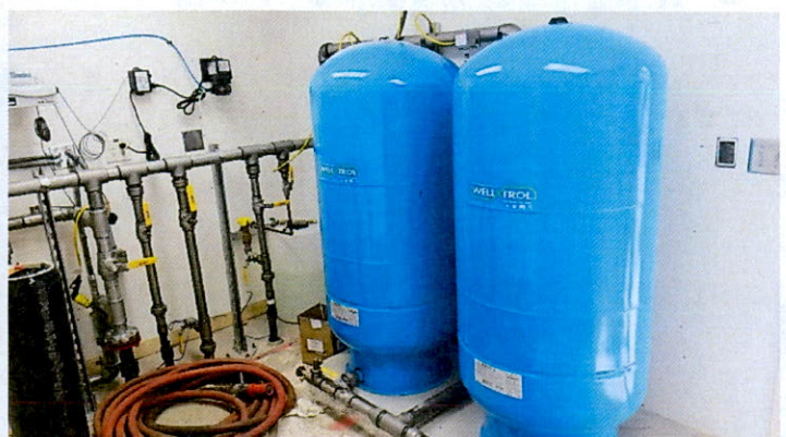
Pump house plumbing and controls
