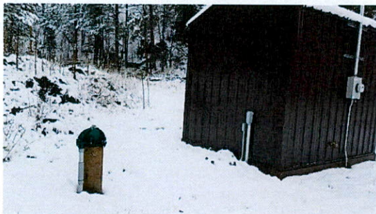
Well # 5 and pump house
