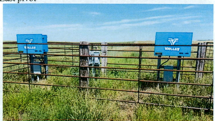
Twin controllers located at junction of 10" and 12" pipelines
