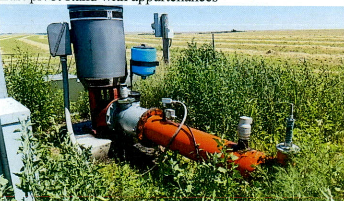
1,800 gpm well with chemigation valve
