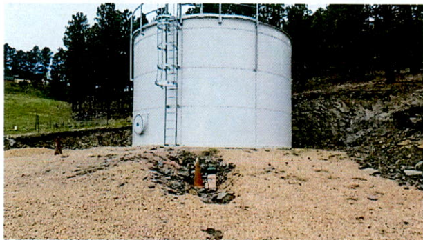
Well in foreground and 50,000 gallon storage
