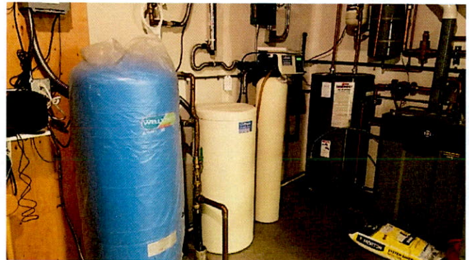
Pressure system and piping
