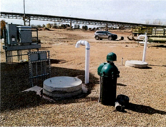
Well with controls and cistern with manhole at each end.
