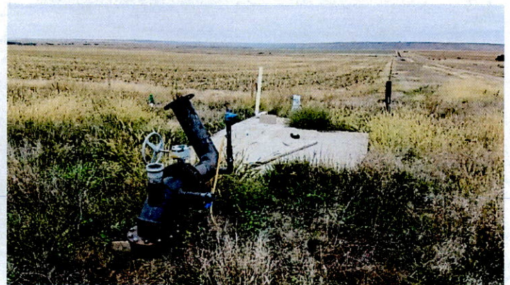
Supply appurtenances for subsurface drip system at pad installed for sand filters
