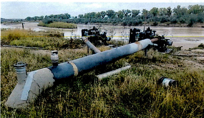
Pump installation on White River
