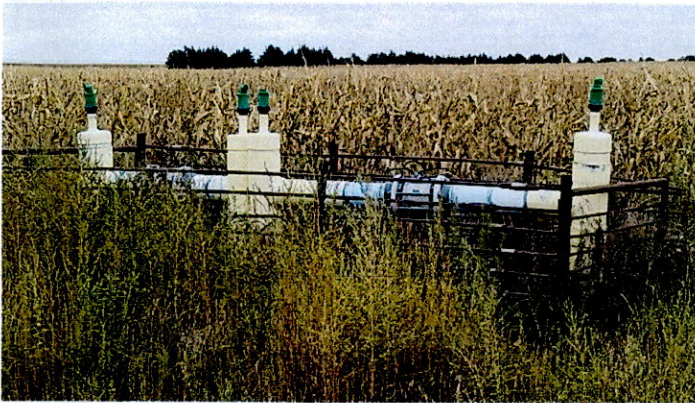
Subsurface system control valves
