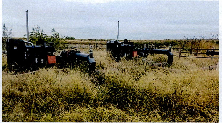
Diesel pump station supplying pivots Pump station supplying subsurface acres removed (far right)
