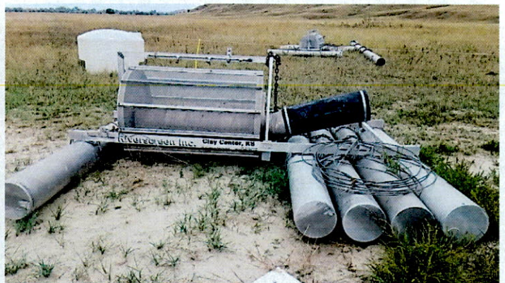
Floating pump intake and trash screen
