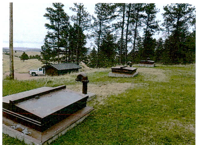
Underground reservoirs of 14,800, 25,940, 24,840 gal.
