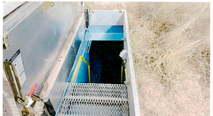
Booster station access
