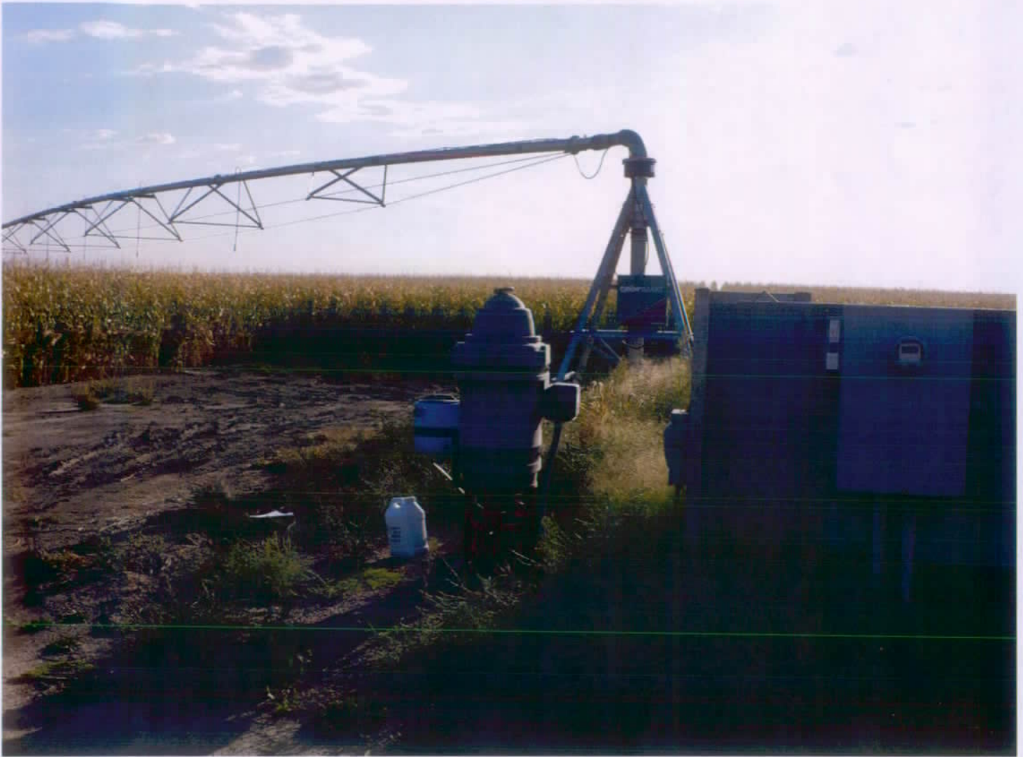
Well head and Pivot center for Water Permit No. 2619-2, Tom O. Milligan
